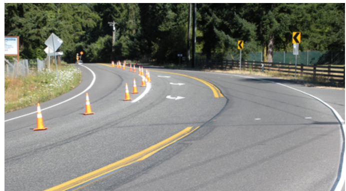
This is the site of the Thurston County demo using county staff, before treatment. A photo of the curve after treatment is above, left.
