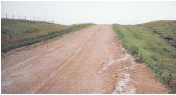
Fig 4. High shoulder causes erosion along edge of road.
