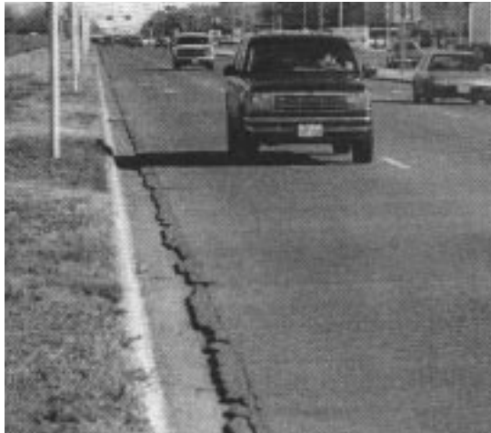
Surface irregularities that run parallel to travel are particularly hazardous to bicyclists.
