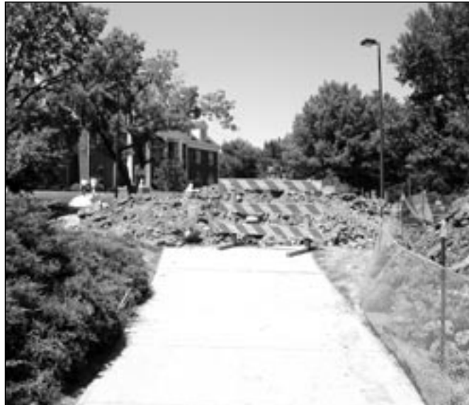
A pile of dirt blocks this sidewalk just before an intersection, forcing pedestrians onto a busy street with no shoulders.
