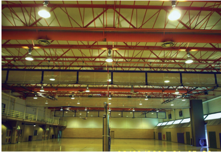
BEFORE lighting upgrade
